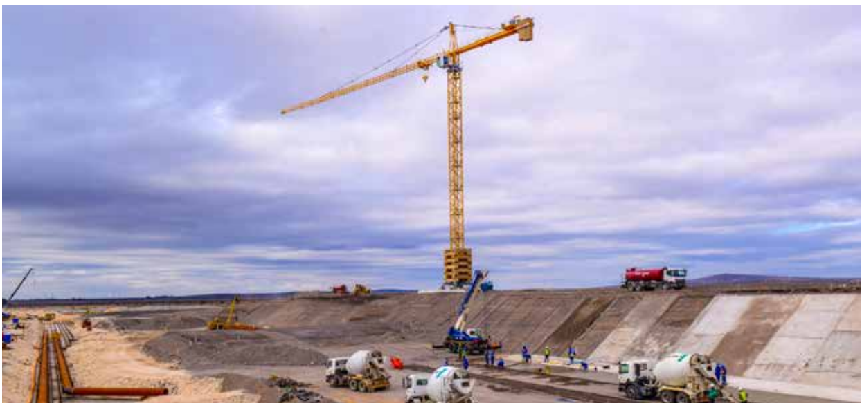
Construction of eight crude oil storage tanks, with a capacity of 1.1 million barrels each, has begun in the Port of Saldanha, Western Cape.
